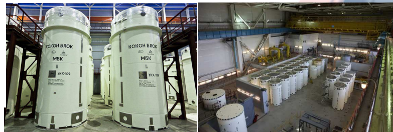
Cask type interim storage facility
